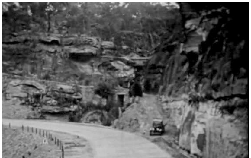
In 1929, a vehicle is seen descending from the Devil's Elbow to the Pacific Highway below. The old road was used to provide access to the construction of the new one.
